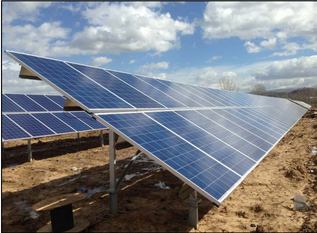
1.5 MWp solar electric system developed by Upsolar in Kozani, Greece.
