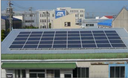
48 kW PV system in Anjo, Japan, using Upsolar smart modules, optimized by Tigo Energy
