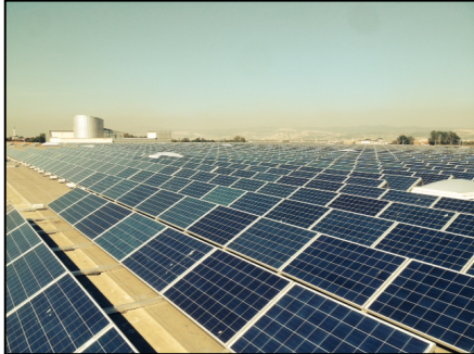
Upsolar's UP-M250P modules power a 650-kWp array for Winsa in Kocaeli, Turkey.
