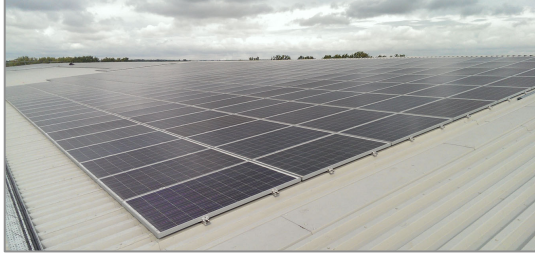
309 kWp rooftop array featuring Upsolar modules, completed in partnership with Photon Energy
